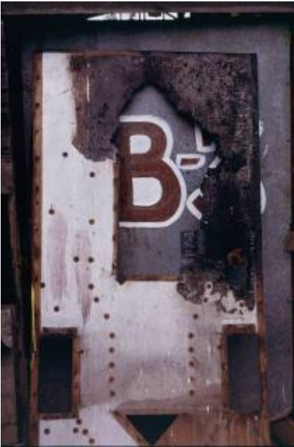
Figure 29: Side wall of a re-circulating batch dryer that caught fire
